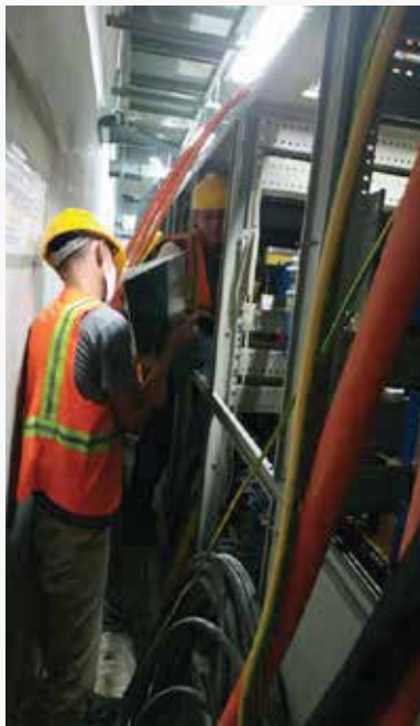
Busbar Connection Check
